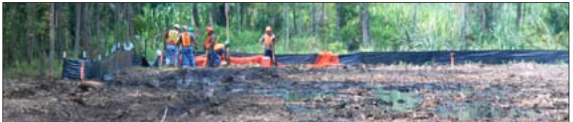
Workers install silt fencing to protect the marshland by providing erosion control.
