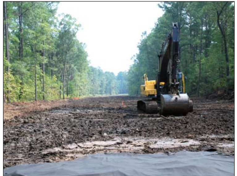
Work began in August on the widening of US 17 in Beaufort County. The project will improve safety while preserving the environment.
