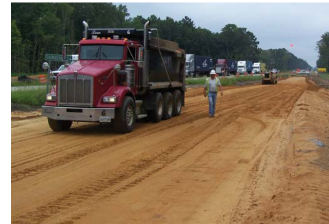
Building new roadway requires a lot of earth moving. This dump truck carries fill material which will be placed layer by layer to create a stable and smooth road bed.
