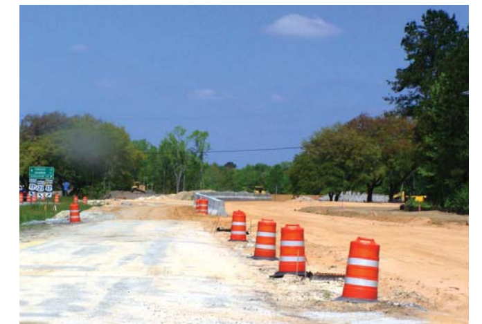
The old northbound lanes of US 21 are being widened to become a new ramp from US 21 to northbound US 17 and a new lane from US 21, under the US 17 overpass, to a roundabout before joining US 17 southbound. This photo shows how the old lanes will split into a new northbound ramp (right side of new barrier wall) and a new travel lane (left side of the barrier wall).
