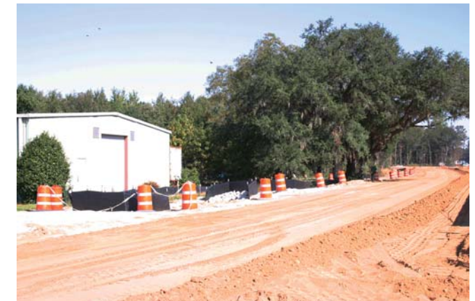
The sub-grade is completed for a new frontage road west of the Gardens Corner interchange. Over the next few months, crews will complete the cul-de-sac and final grading before placing asphalt.
