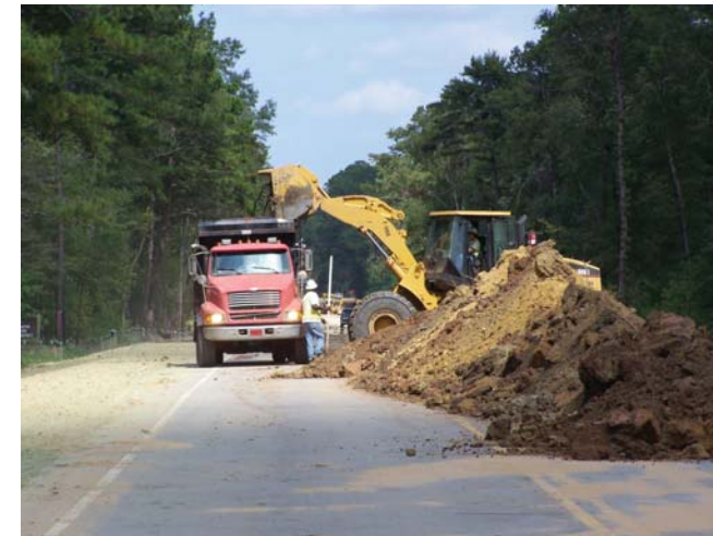
Crews excavate dirt along the edges of the existing US 17 roadway to widen the shoulders for what will become the new northbound lanes. The widened roadway on the left side of the picture begins to show how much safer the new shoulders will be.
