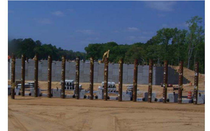
At the Gardens Corner Interchange, the southern MSE wall for the new US 17 overpass has reached its final height and construction of the northern MSE wall is now underway.
