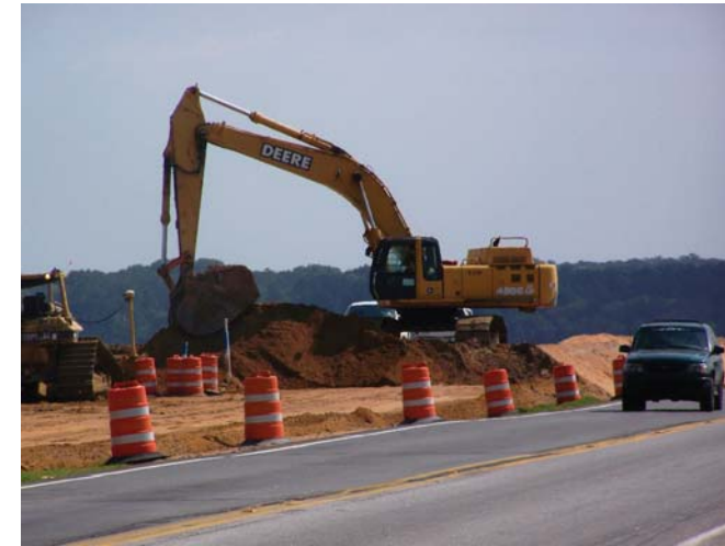
After installing approximately 10 lifts of surcharge material on the Segment 2A causeway, just north of the Harriet Tubman Bridge, much of the foundation is now compact enough to begin removal of the surcharge. A track hoe removes surcharge material from Segment 2A.
