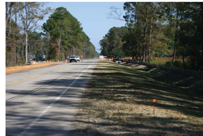
Work on the old roadway between the Combahee River and Big Estate Road includes wider paved and landscaped shoulders.
