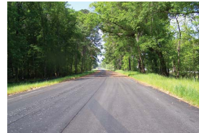
Binder and surface course have been placed on the northbound lanes between the Harriet Tubman Bridge and Jacob White Road.
