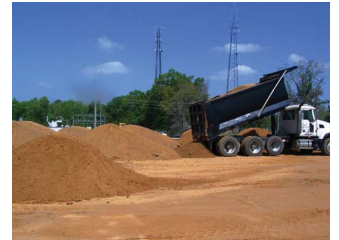
Surcharge material removed from Segment 2A, north of the Harriet Tubman Bridge, is used as fill for the 20' high embankment supporting the approaches to the new US 17 overpass at the Gardens Corner Interchange.
