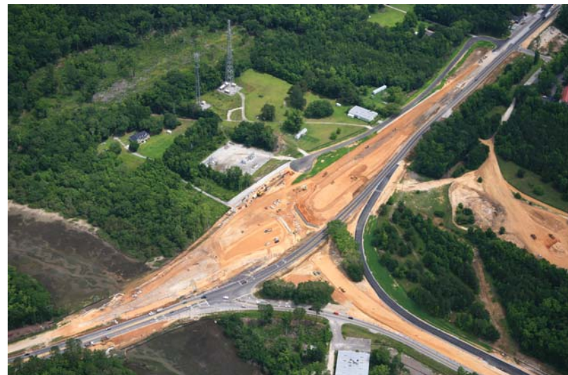
Aerial photo of the US 17/21 Gardens Corner Interchange. (Frontage Road, southern MSE wall and pile cap, and much of Ramp 1 are complete. The northern MSE wall and pile cap, Ramps 2, 3, & 4, US 17, and US 21 are all underway.)
